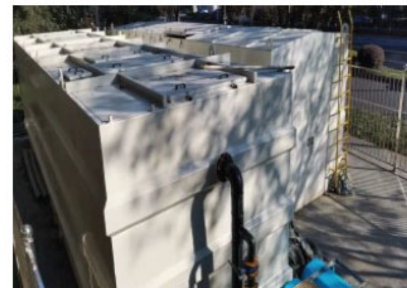
CMFF skid on customer's site
