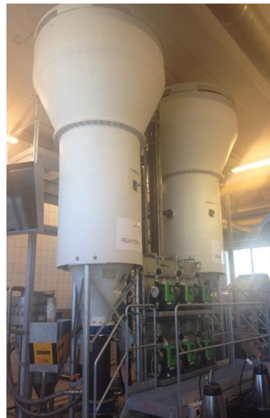
Figure 1 - Struvite reactors, Aaby WWTP
