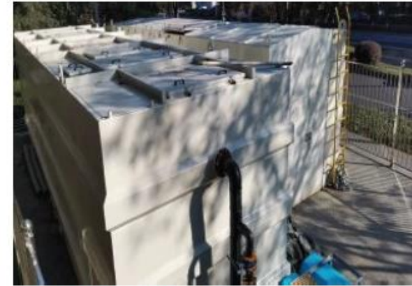
CMFF skid on customer's site
