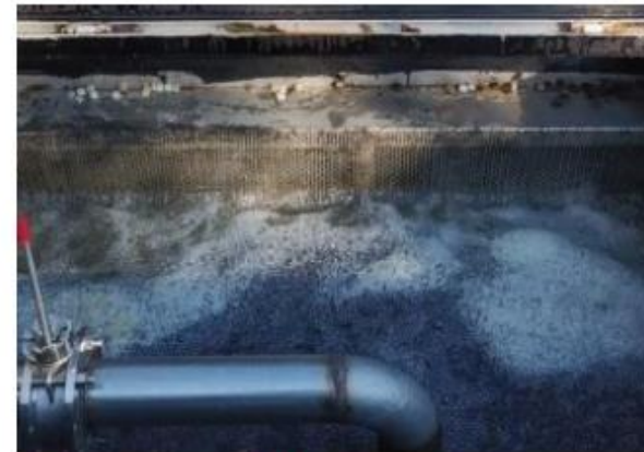
Carriers in aeration stage
